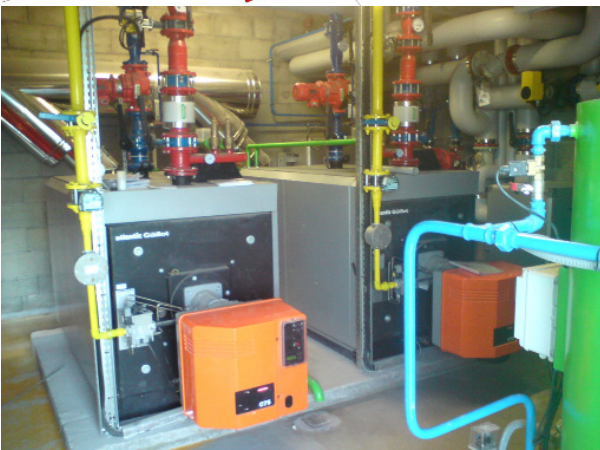
A virtual project and the production of the boiler room of the "Quartier Colbert" project in Nevers.
